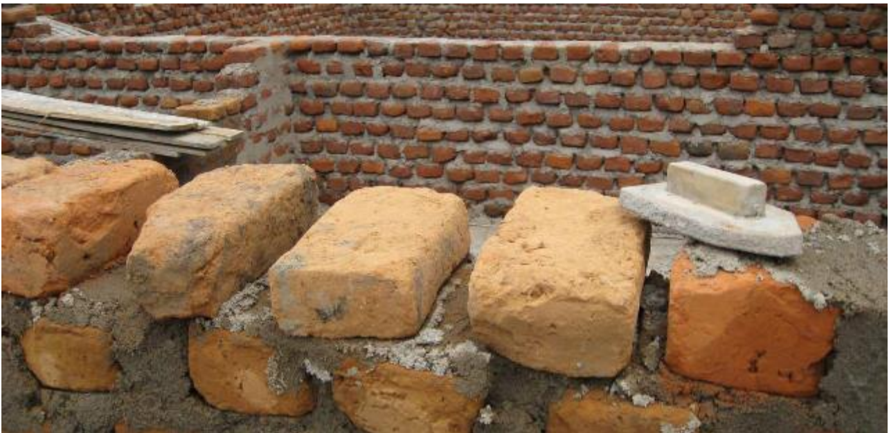
New school being built in Moliandru Village. Photo credit: BBC World Service/Flickr.com/ CC BY-NC 2.0
