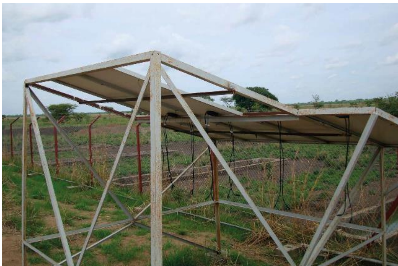
Solar panel at Abiriu Haffir. Photo credit: Arshad Khan, UN Environment
