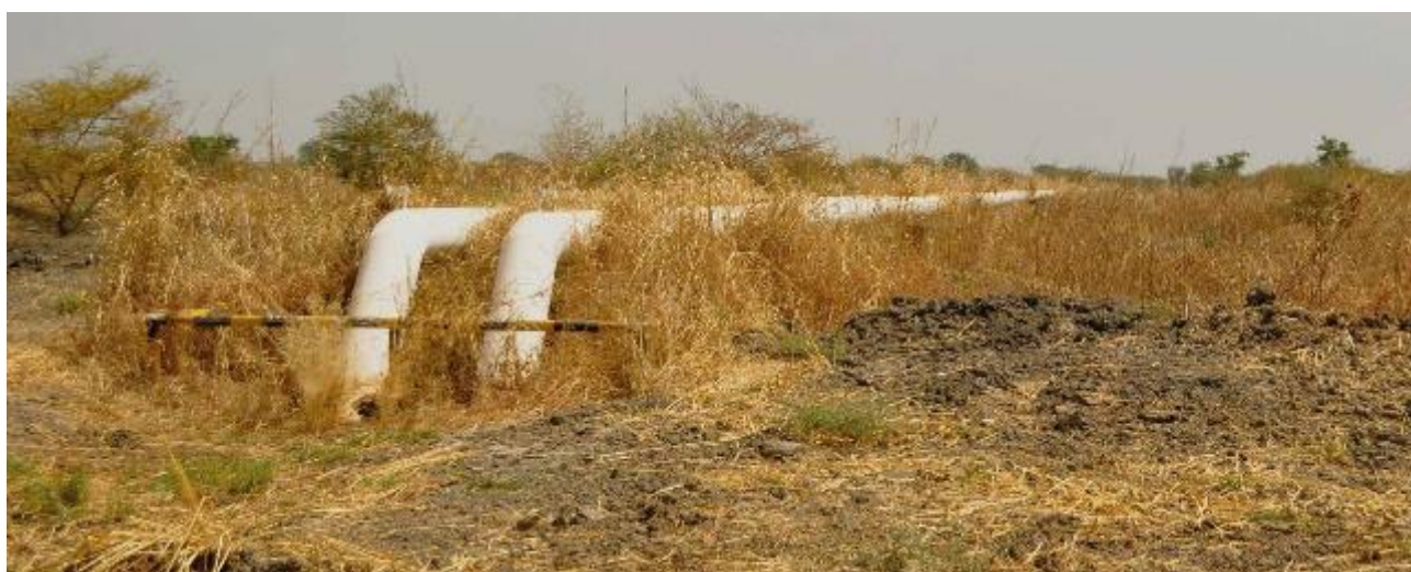
Oil pipeline on the road from Bentiu to Yida. Photo credit: Shannon Orcutt/ Flickr.com/CC BY-NC-ND 2.0
