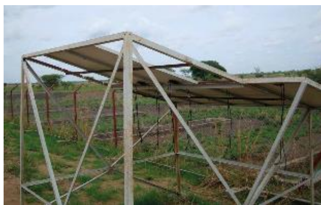
Solar panel at Abiriu Haffir. Photo credit: Arshad Khan, UN Environment
